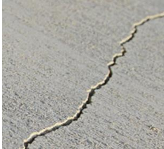
Figure 5: Drying Shrinkage Crack (SCP file photo)
