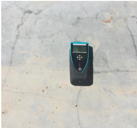
Figure 2: Plastic Settlement Cracks (SCP file photo)
