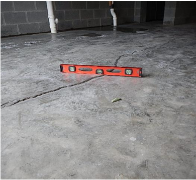
Figure 4: Settlement Cracking (SCP file photo)
