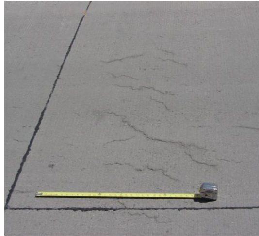
Figure 1: Plastic Shrinkage Cracks (image from ForConstructionPros.com)
